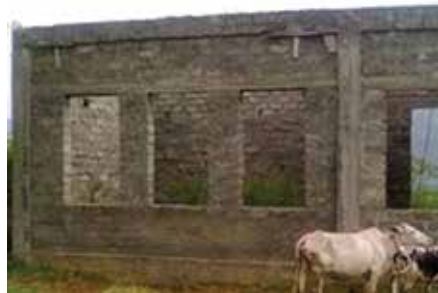
Incomplete school of Village Kolay
